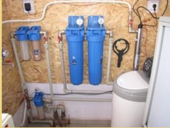
LWW System installed in Reformed Church Nursing Home -- 2011
